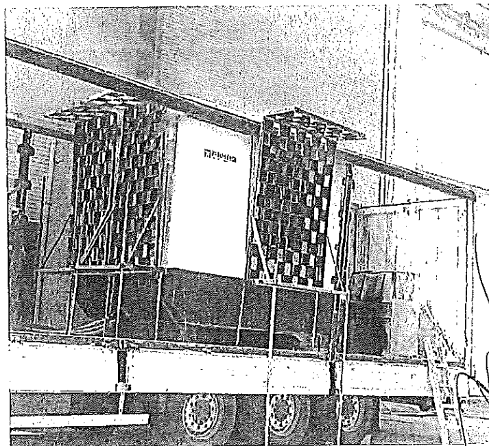
Photos 4 – Aspect of 20/0.4 kV, 800 kVA Concrete Substation in test circuit after internal arc test for IAC-B
